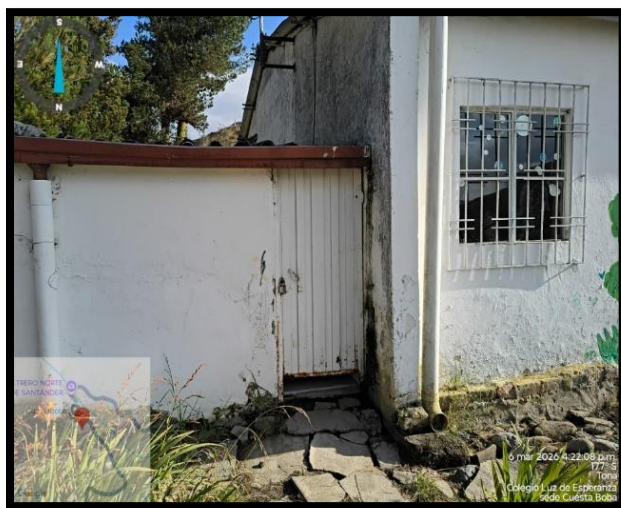
Figura 43. Riesgo peatonal inestable
