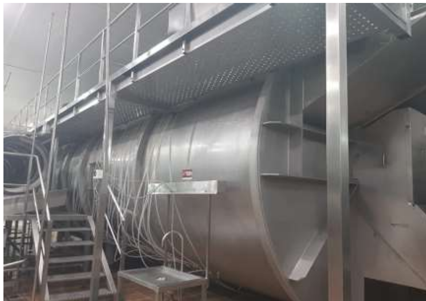
Figura 1. Chiller, pre 1 y pre 2
